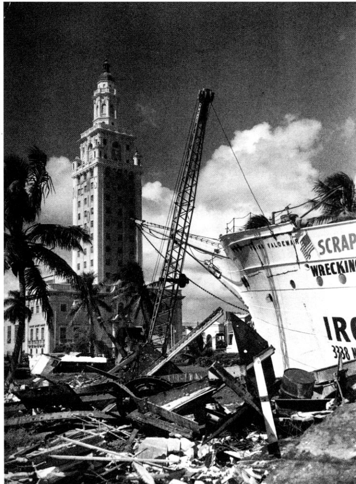
Left— The Prins Valdemar was converted into the Miami Aquarium in 1928. The public could view up close alligators, tropical fish, sharks, turtles, piranhas, octopuses and iguanas. HMSF 1996-421-11. Above—Declared structurally unsound, wrecking crews dismantle the vessel, December 1952. HMSF, Miami News Collection 1989-011-150057.
